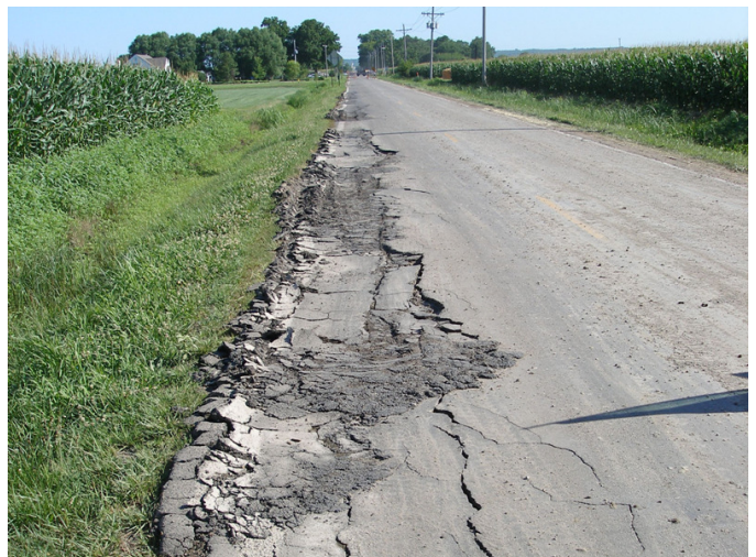
Pavement damage Route 9
